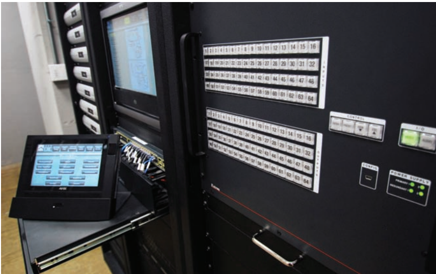
The 64x64 Extron Cat-5 switcher, which routes any signal from any source to any combination of displays and sound systems in the facility.
